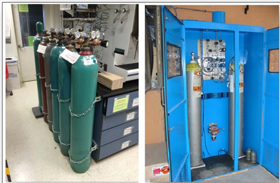
Figure 3.15: Gas Cylinder Storage
