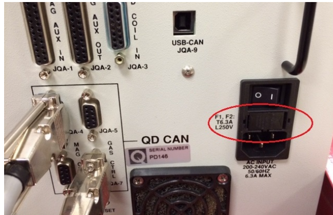
Figure 3-6. Location of the two, paired delay fuses (6A, 20mm) at the CAN tower power entry
